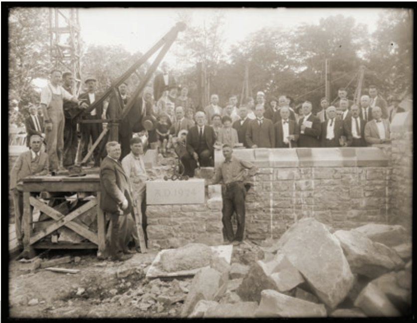
Laying the cornerstone of the college’s new administration building on September 4, 1924. Later named Holland Hall, the building remains one of St. Olaf’s most iconic structures. ST. OLAF COLLEGE ARCHIVES
